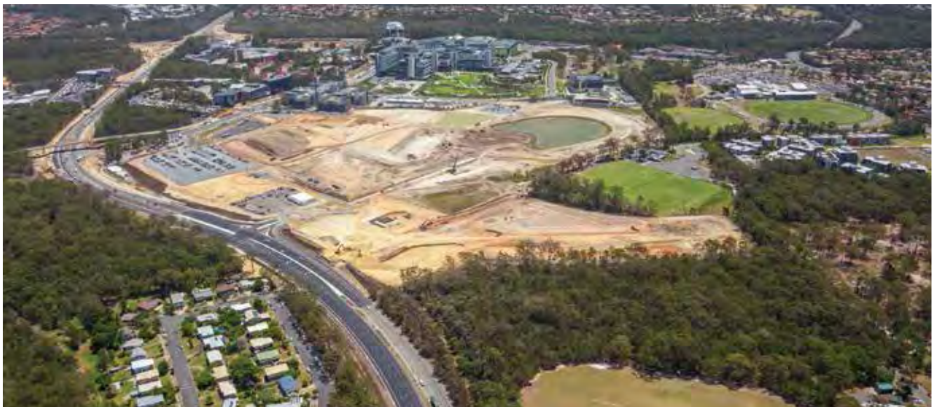
Smith Street Motorway upgrade and construction underway on the Gold Coast 2018 Commonwealth Games Athletes Village
